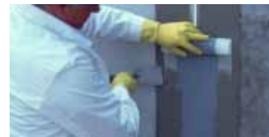
2 Place VANDEX DILA JOINT TAPE, followed by working fabric edges on both sides into waterproofing slurry.
