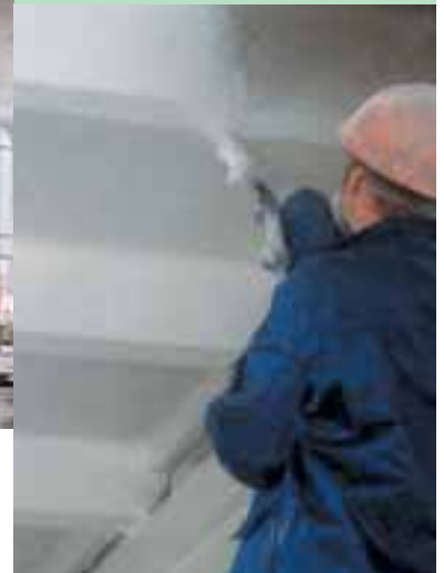
Water treatment plant at the Kurjanovo Aeration Station, the largest in Europe, in the process of refurbishment.
